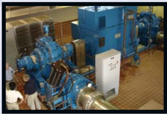
◀ Figure 5. 3,500 HP Pump Being Monitored by CBMi
